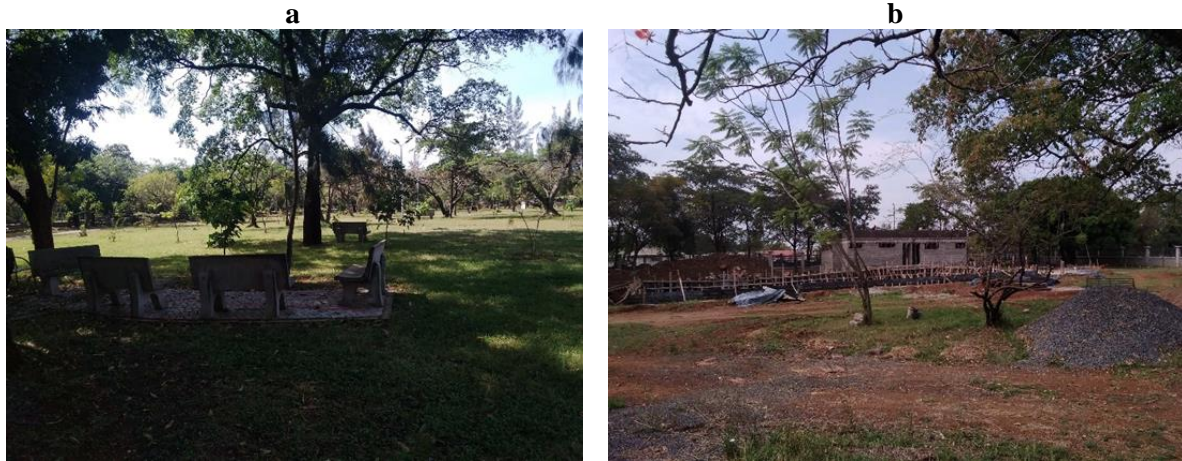
Plate 8: a) new concrete seats, b) Ongoing works on the swimming pool and changing rooms
